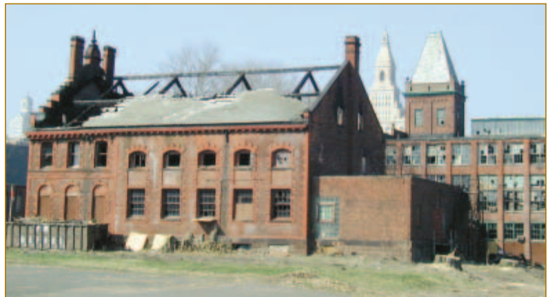
View of former Capewell Horse Nail Company administration building on Governor Street, showing fire-damaged roof.
