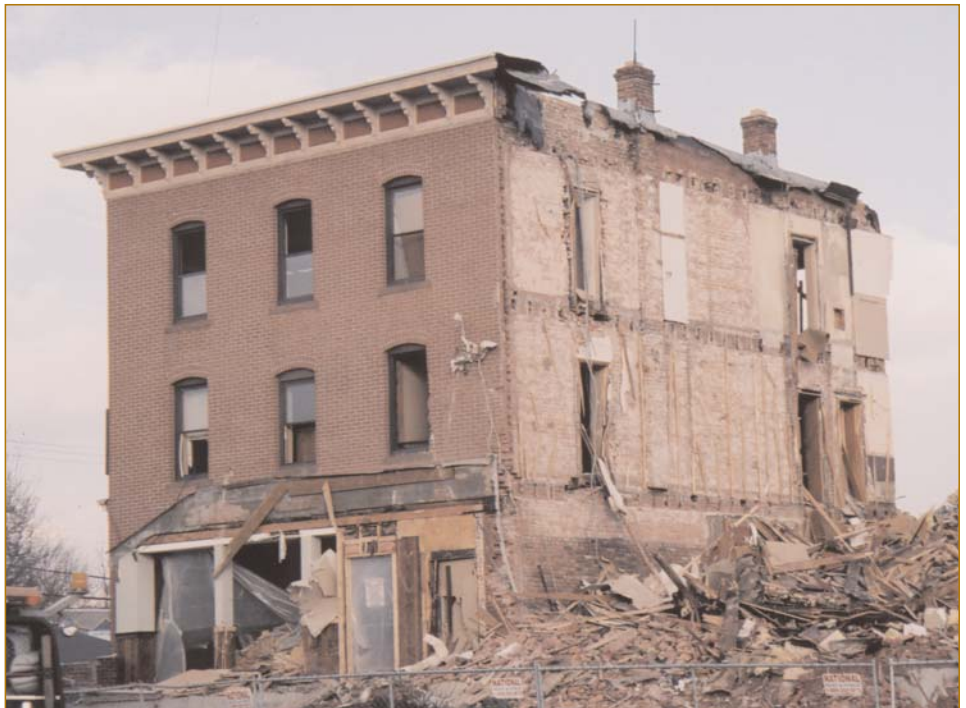
The partially demolished Carmichael's Restaurant at Wethersfield Avenue and Airport Road. Photo: Rafie Podolsky.
