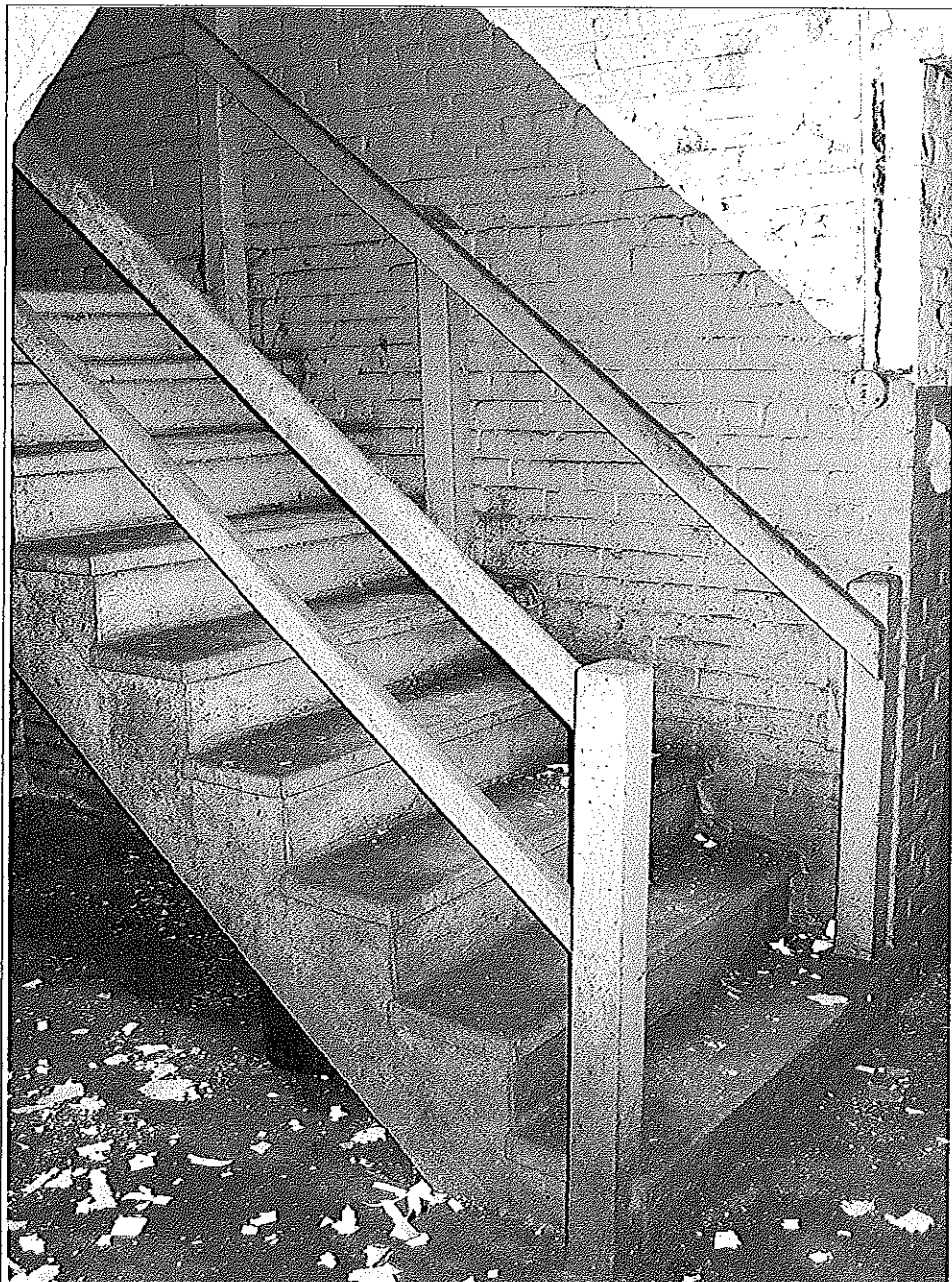
Photograph 14: Detail of main stairway in original part of factory, camera facing south.
